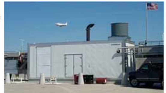
A prepackaged cogeneration plant at Greater Rochester Airport, New York State. This enclosure is home to a 750 kW natural gasfired Waukesha synchronous generator with full engine and exhaust heat recovery. These units normally run parallel with the utility, but kept the airport fully functional during the great blackout of 2003. Waste heat is used for both building heating and driving a 300-tonne hot water absorption chiller
