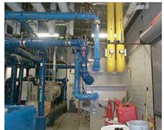
A large absorption chiller using cogen waste heat provides 250 tonnes of cooling to a large high school
