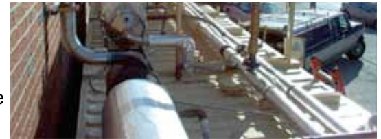
Exhaust heat-recovery exchangers and catalytic converters, mounted on the roof of a prefabricated enclosure of a packaged 380 kW modular system at 4C Foods in Brooklyn, New York. A standard container can be trucked across the US without special permits. Sound is attenuated to less than 45 dB at 6 feet (1.8 m)
